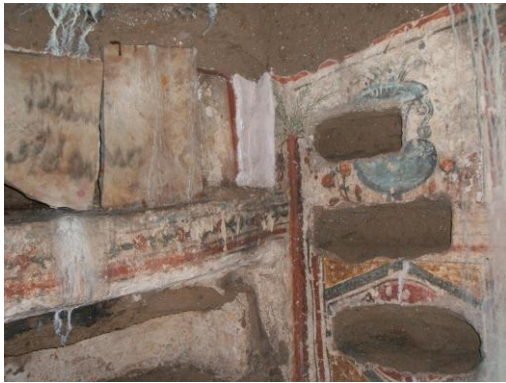
Figure 3. Cubiculum in the Vigna Randanini catacomb, showing damage from water and the scribbling in charcoal over some of the tombs.
